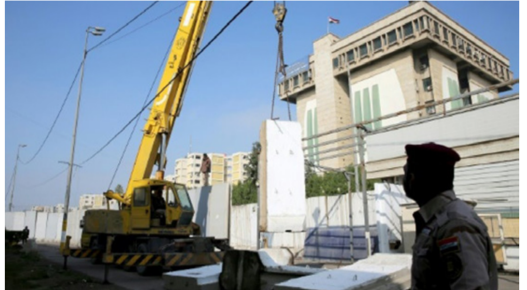
Workers remove cement blast walls surrounding the Iraqi foreign ministry near Baghdad's Green Zone
